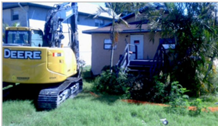
This abandoned house on SE 3rd Street in Belle Glade is one of 70 structures targeted for removal.
