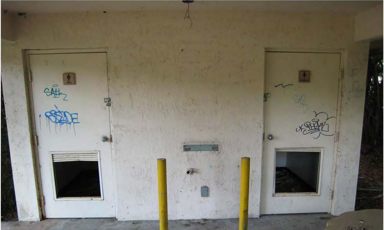
Examples of Vandalism
