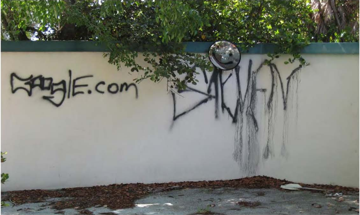
Examples of Vandalism
