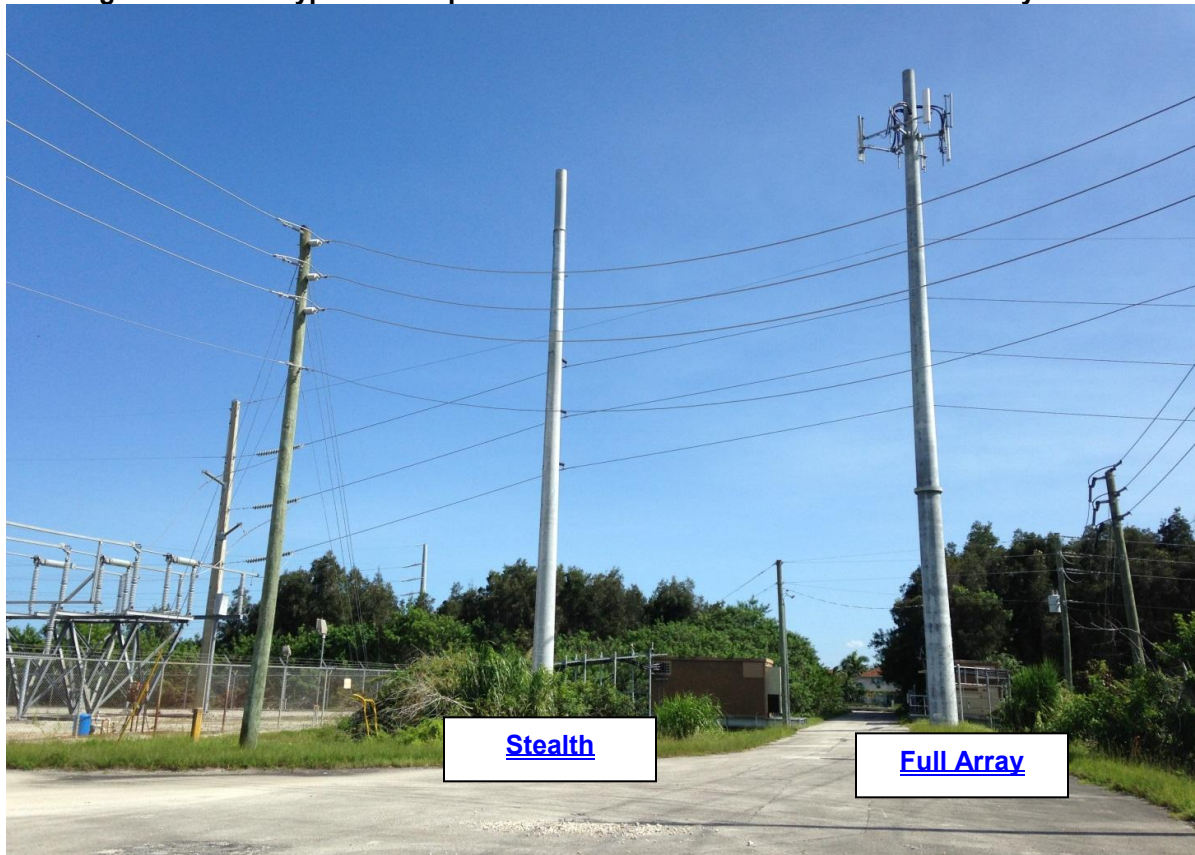
Figure 4.B.9.D - Typical Examples of Electrical Transmission Poles or Utility Structures
