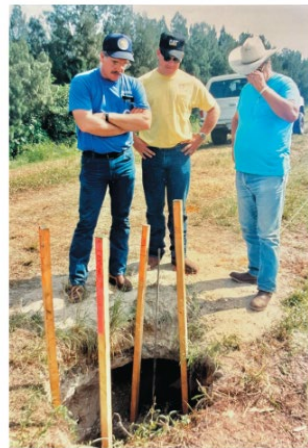
Figure 7. Sink hole on landside slope that developed during 1995 high-water event.
