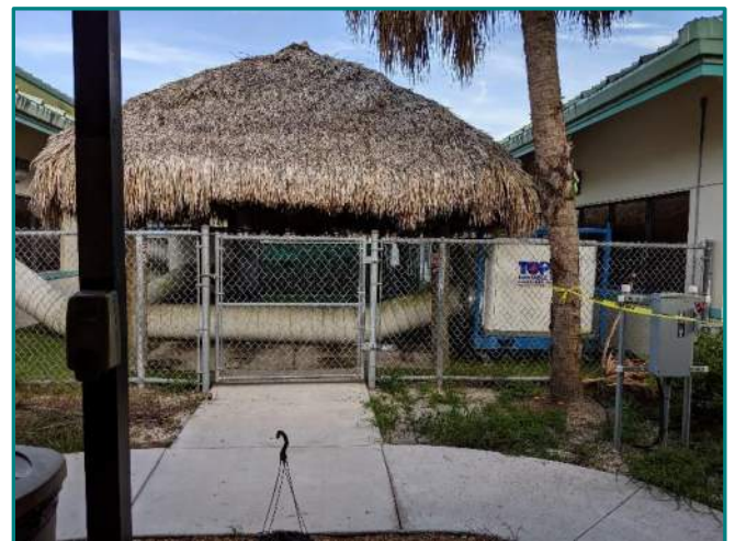
9 Play yard with air conditioning duct work
