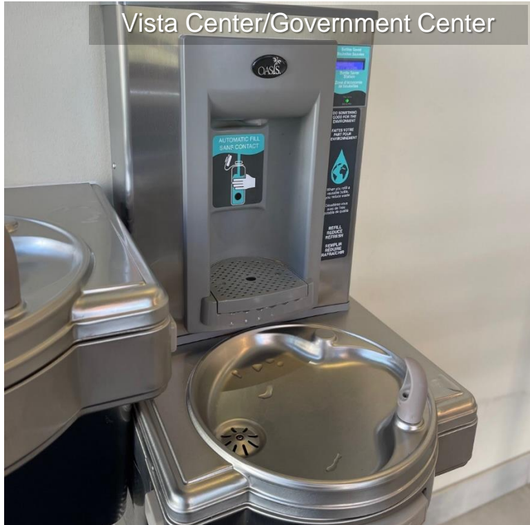
19 touchless water refill stations installed
