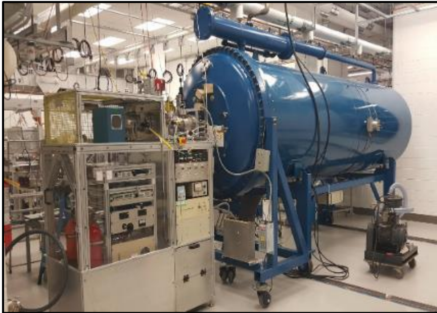
Ion source & Accelerator
