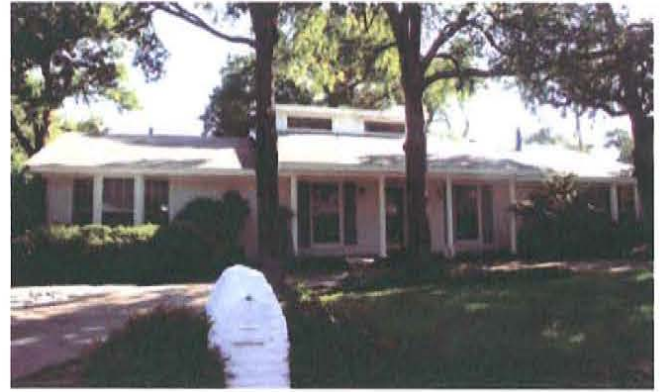
Figure 68. Ranch house in Arlington, Texas, constructed c.1965, with a modern shed dormer that alters the roofline and results in diminished integrity; it is considered not individually eligible (Mead & Hunt photograph).
