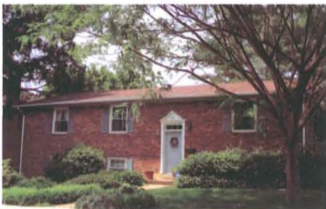
Figure 26. Split-foyer house in Arlington County, Virginia, retains its original form but features only one architectural element: applied Colonial Revival details. As a result, it does not meet the survey criteria (Mead & Hunt photograph).
