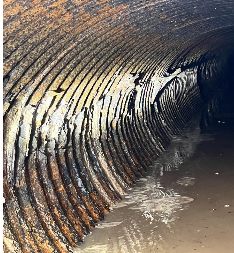
CMP spring line failing weakening pipe structural integrity
