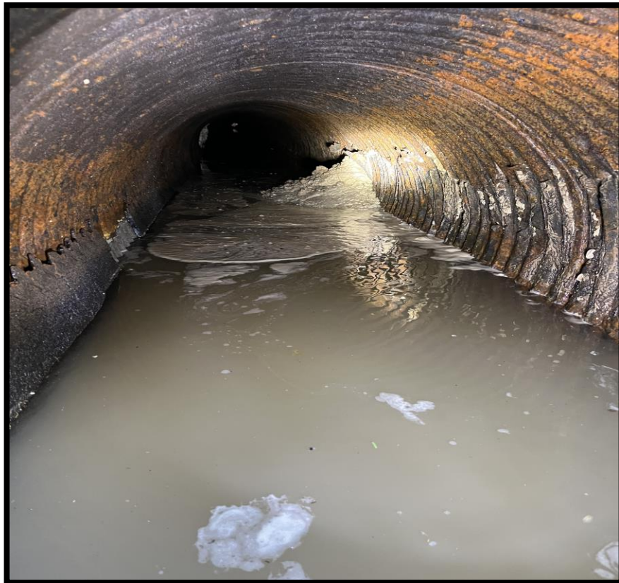
CMP spring line section loss
