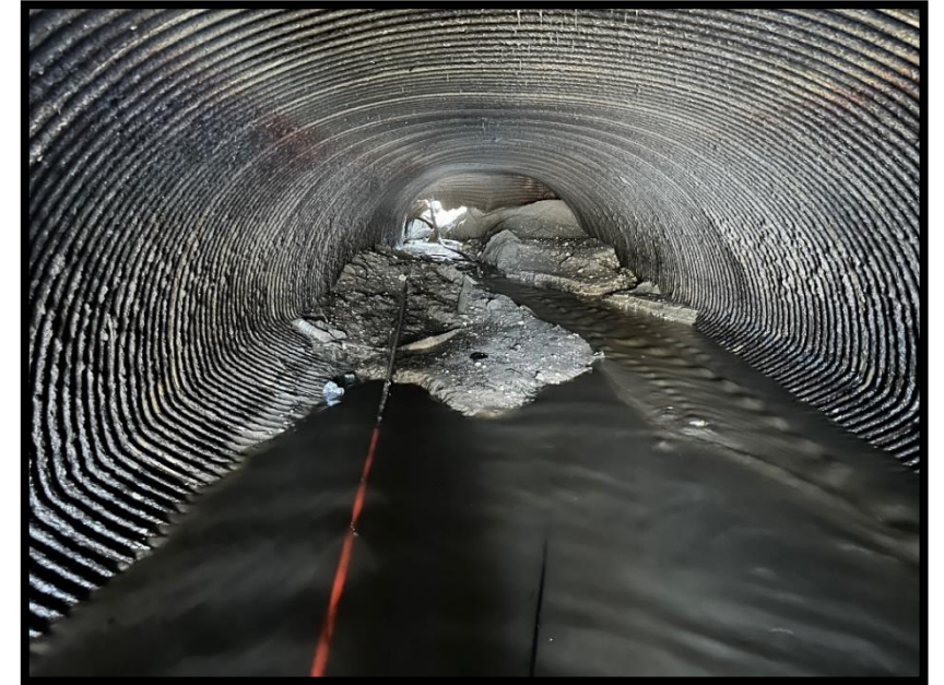
CMP failure – collapse / blockage
