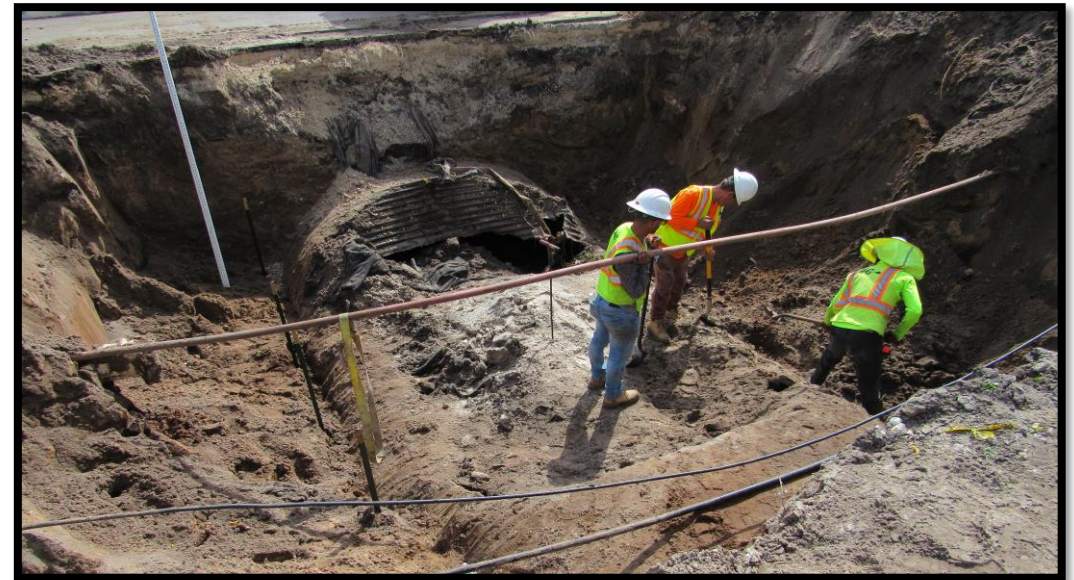
Collapsed CMP sinkhole
