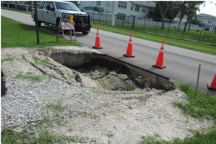
CMP failure - sinkhole
