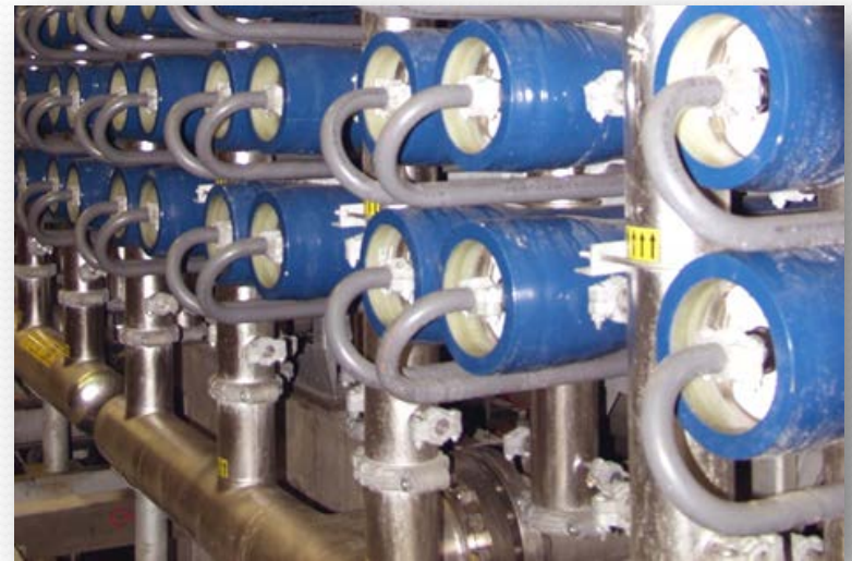
Desalination membranes at Tampa Bay Water's plant.
